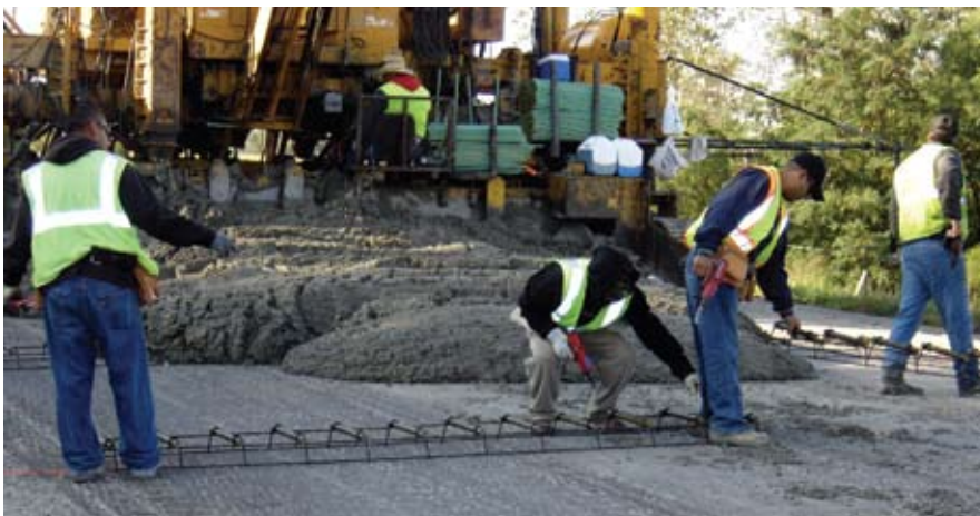
A crew from Manatt’s places a concrete overlay on U.S. 71 in Montgomery County, Iowa.
