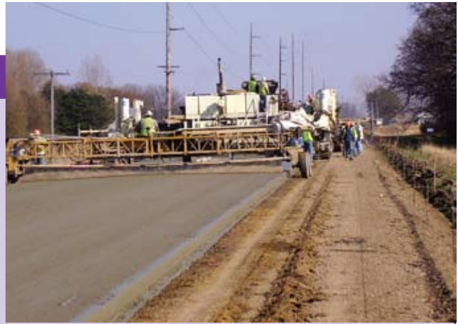
This concrete overlay was placed over a reclaimed asphalt base in Freeborn County, Minnesota.
